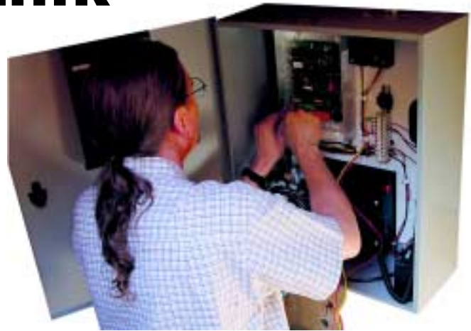
Kimball Communications technician, Ken McGill, puts the finishing touches on a Model 18 installation.
